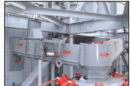
Silo penetration adaptor with flow control valves feeding loadout station.
