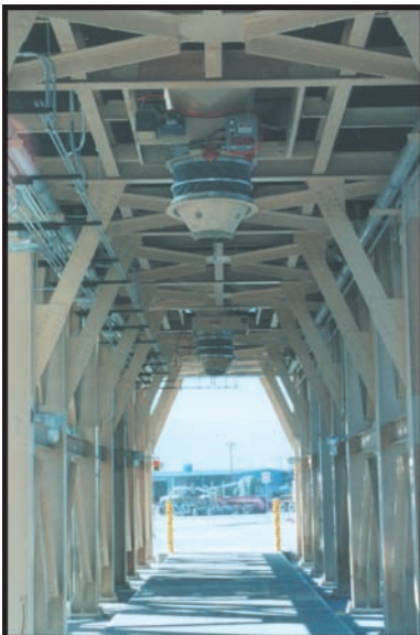
Loadout station equipped with two loading spouts and positioners.
