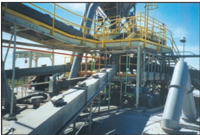
Aeration conveyor run.
