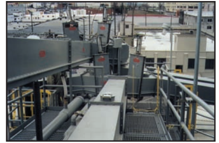
Aeration conveyors distributing to multiple silos using a combination of turning boxes and vertical slide gates.
