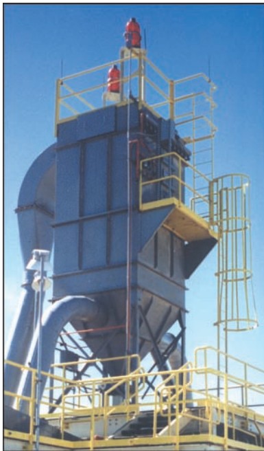
Dust collector with access platform and safety hand rail.
