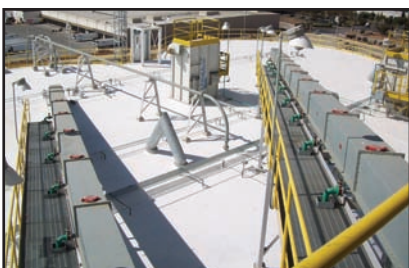
Aeration conveyors feeding multiple silos.
