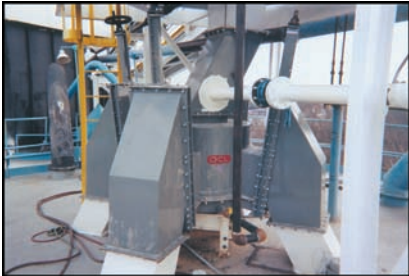
Aerated distribution box with four discharges.
